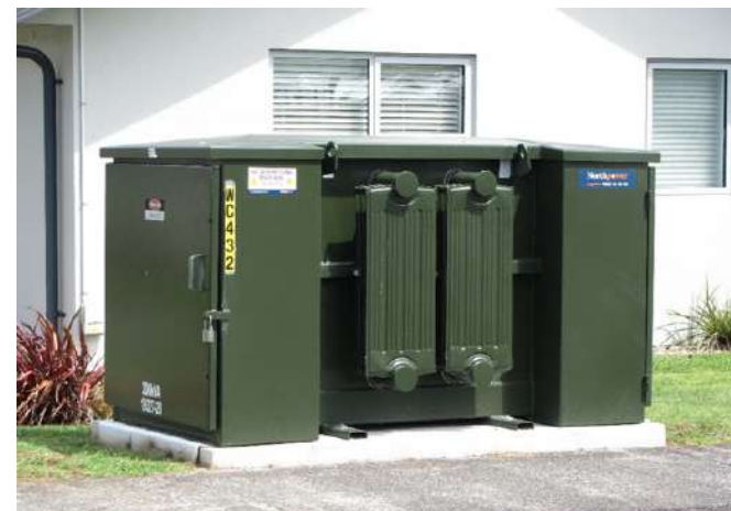
Figure 9.39: Ground-mounted distribution transformer
