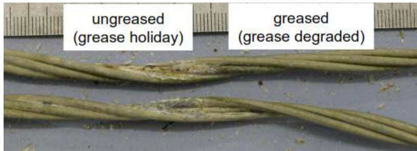
Figure 9.4: Gopher ACSR conductor with grease issues
