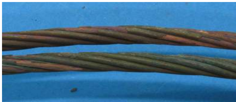
Figure 9.5: Copper conductor sample from a coastal area, showing corrosion
