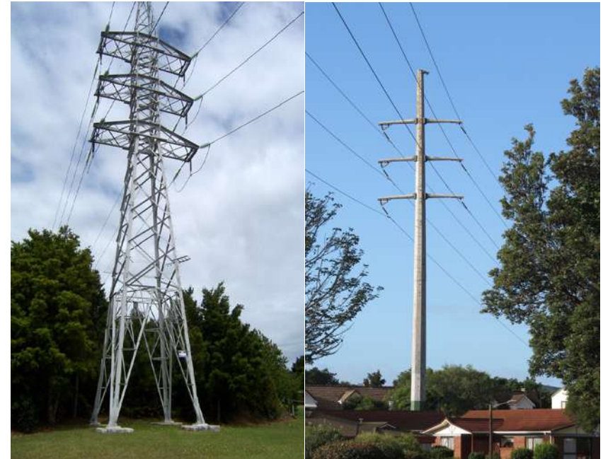
Figure 9.11: Transmission lattice tower (left) and steel monopole structure (right)
