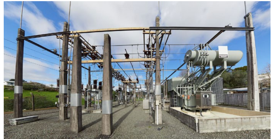
Figure 9.21: Tikipunga zone substation outdoor switchyard
