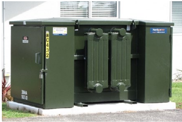
Figure 9.39: Ground-mounted distribution transformer
