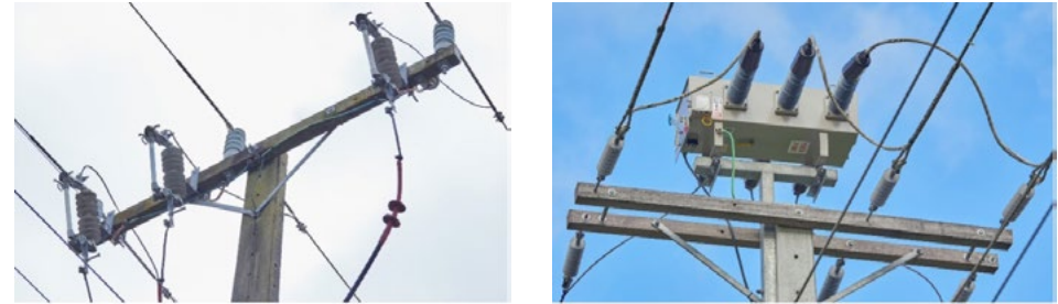
Figure 9.16: Crossarm assembly with drop-down fuses (left) and double crossarm arrangement (right)
